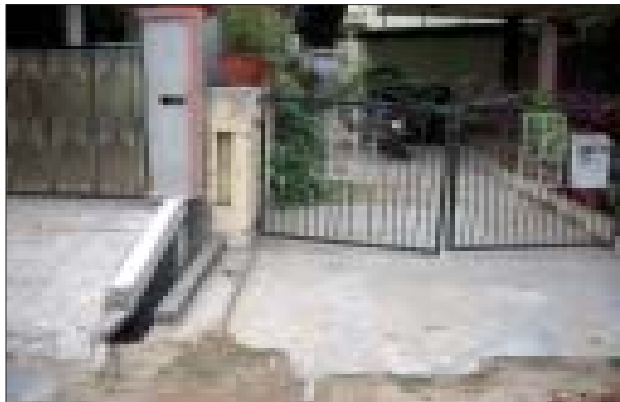
Adjoining homes built on different plinth levels leading to variance in incline of driveways
